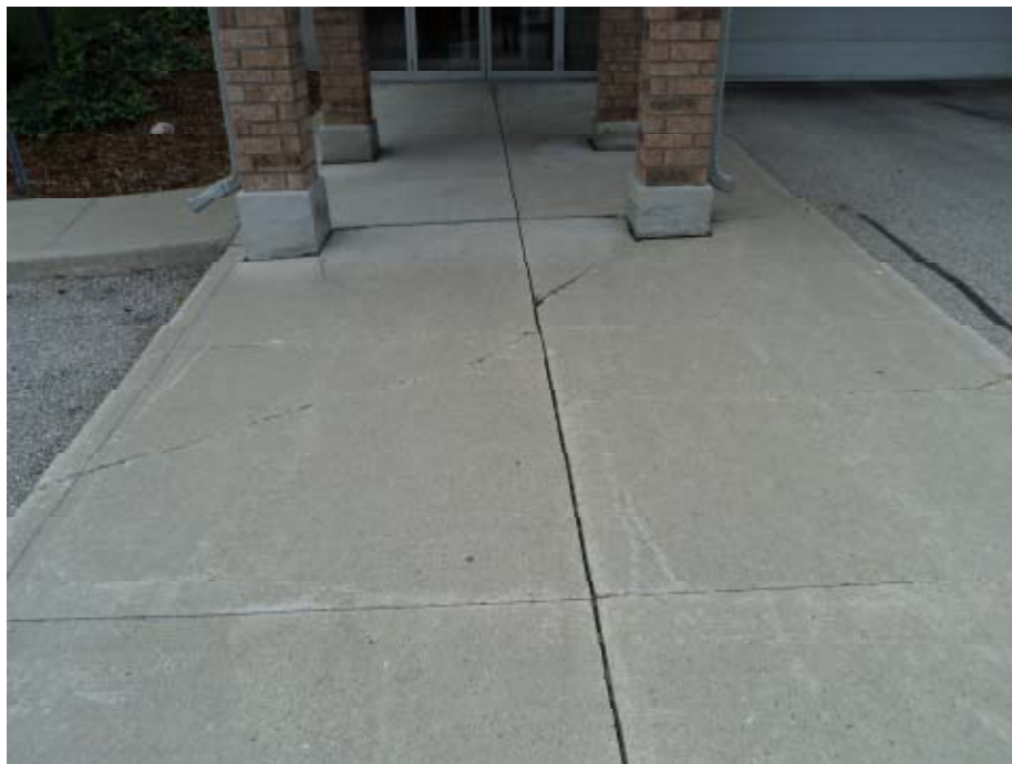
Photo 2 – Main entrance side walk to the complex. Note cracks
