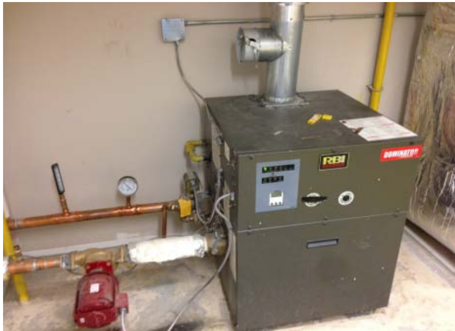
Photo 13 – Boiler located in Mechanical room.
