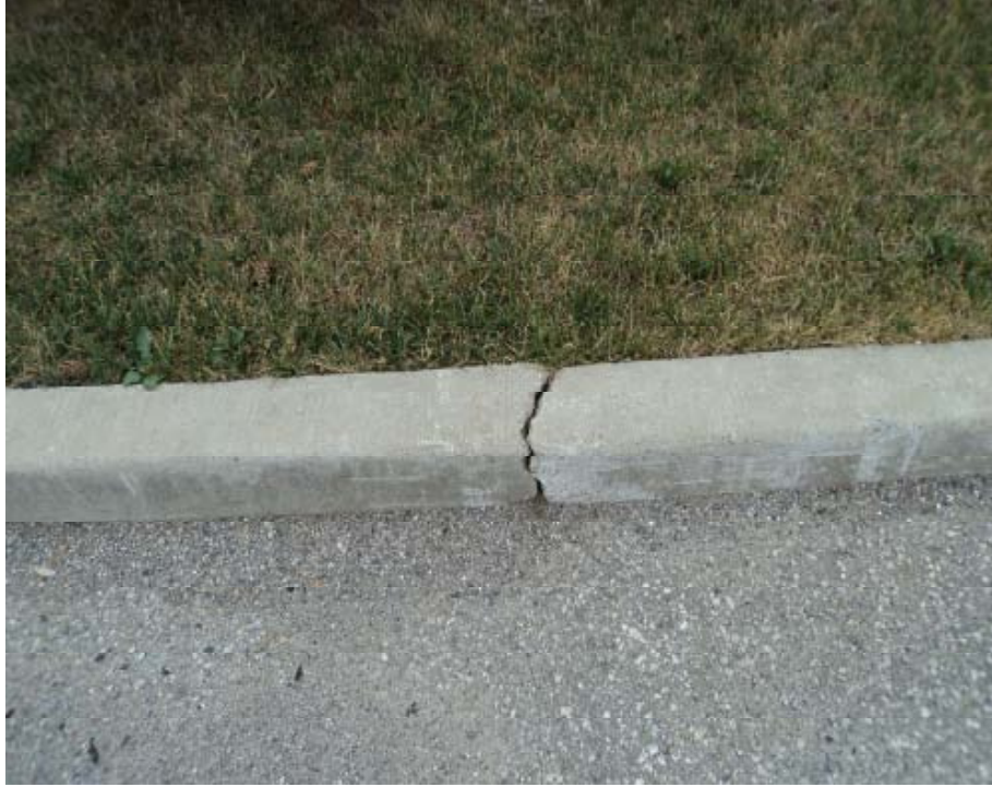
Photo 1 –Cracks in the curb.
