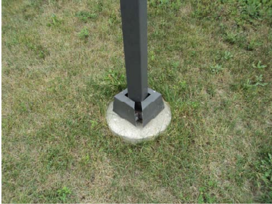
Photo 10 – Parking lot lighting fixture base ajar.
