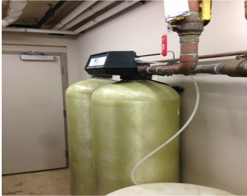
Photo 12 – Two tank water softener
