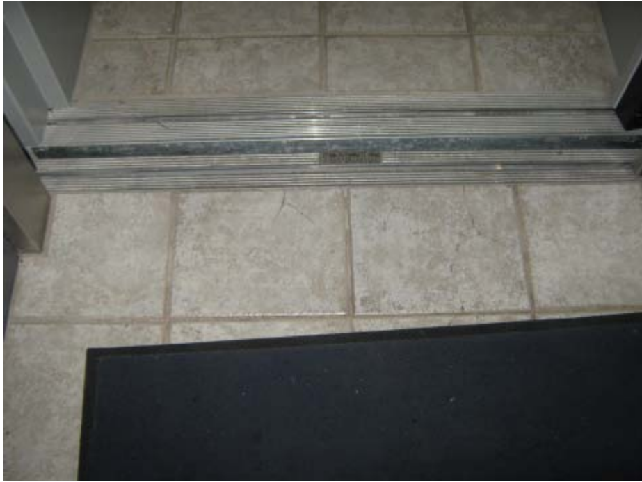
Photo 14 – Cracked ceramic tiles in elevator.
